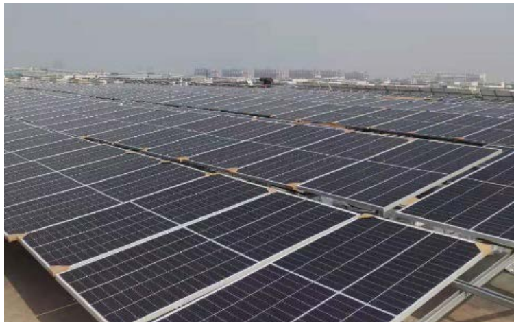
Solar array at Diodes Shanghai Assembly and Test Facility
